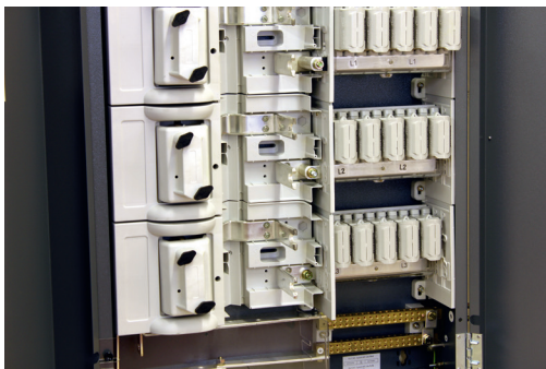
2 J MSDB Shrouds and fuse handles removed from one J way to show cable connection points
