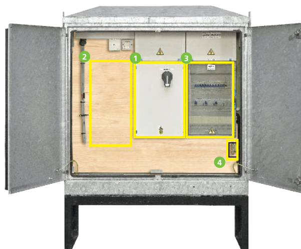
Example of EVIS Pillar for a DNO supply
